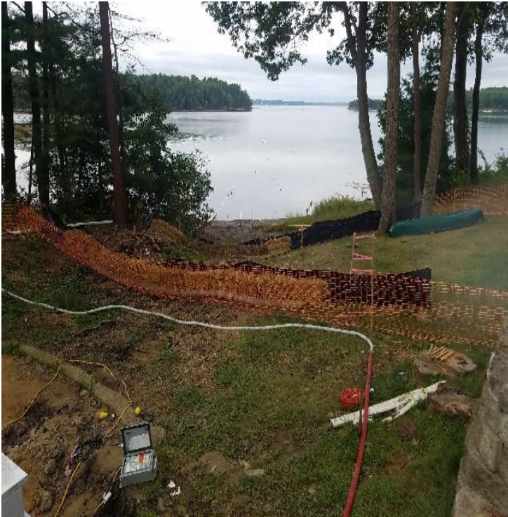
Fig 17: Erosion and sediment controls installed downslope of manhole at Gundalow Landing. Viewing southwest. (9-10-19).
