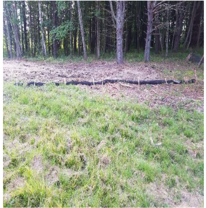
Fig 14: Filter sock installed downslope of where the soils were spread out on the Pickering property. Viewing east. (9-10-19).
