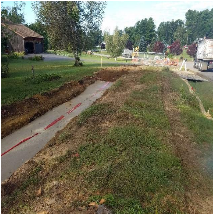
Fig 11: Duct bank along Gundalow Landing Rd. Viewing west. (9-9-19). Rd.
