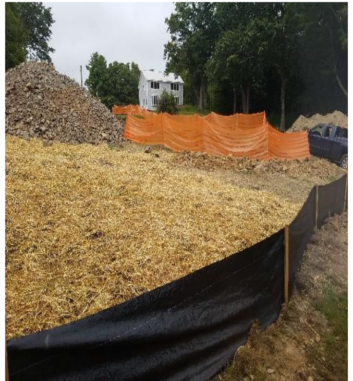
Fig 20: Sediment and erosion controls installed downslope of trenching activities on the west side of the Bay. Viewing west. (9-10-19).
